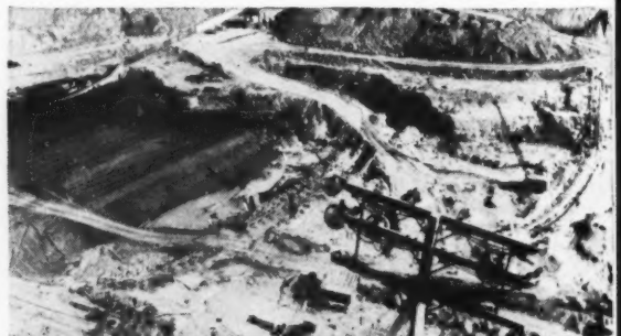
Looking down 300 feet to the coffer-dam construction. A battery of 10 G-E floodlights (Type L-68) in foreground.
